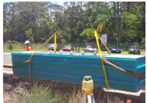
Sunshine coast field test site installation
